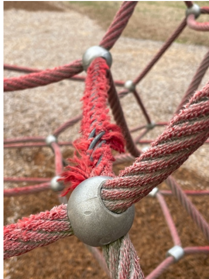
Figure 9 Worn covering on net cables
